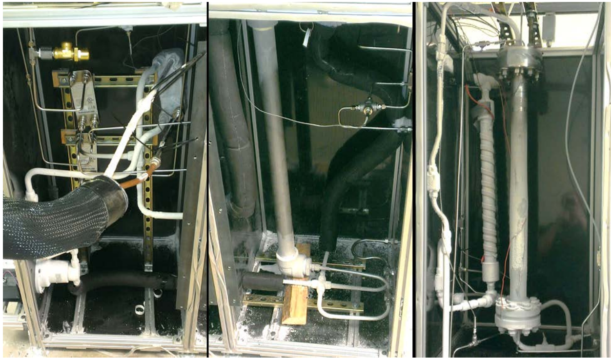
Figure 4-7 Inside view of cold boxes with perlite insulation removed. From left to right: heat exchange and pumping cold box, reservoir cold box, and bubbling heat exchanger and separations cold box
