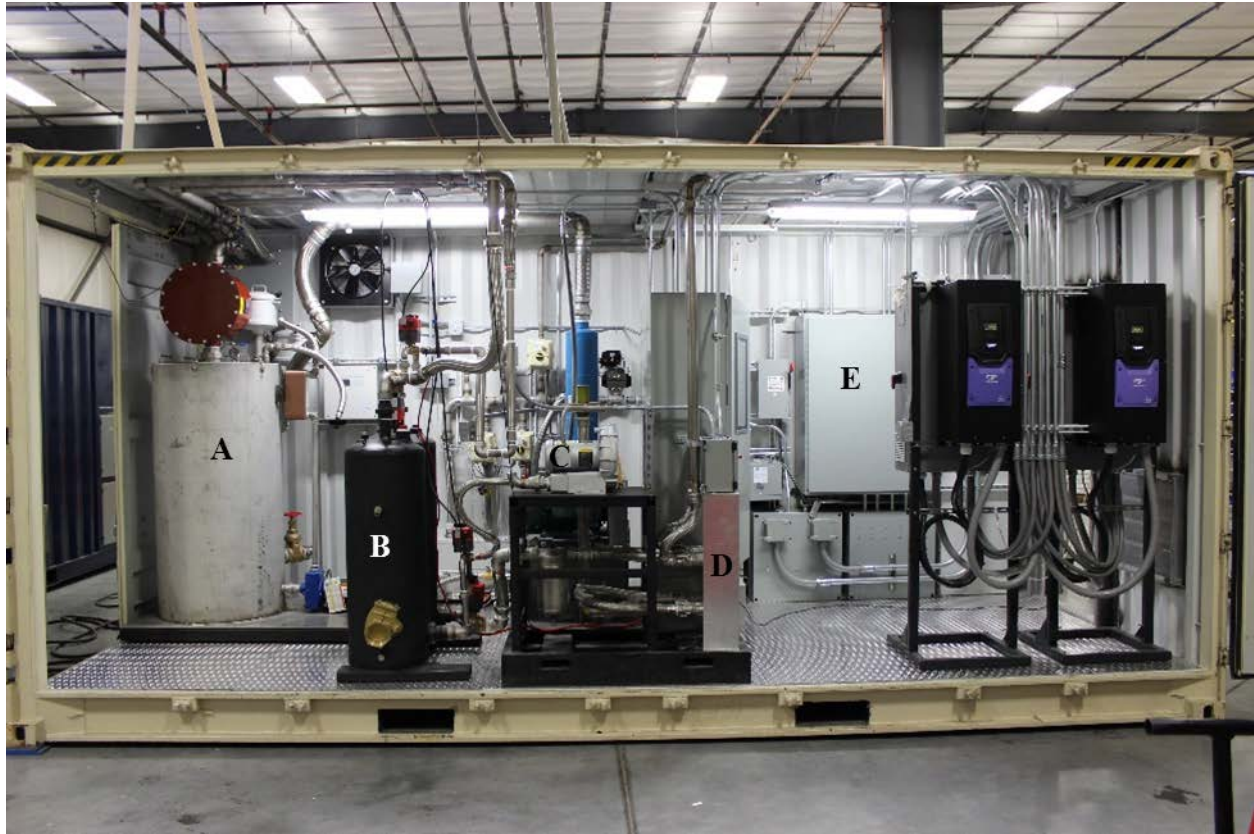
Figure 4-4 Flue gas conditioning skid for CCC ES with deep flue gas desulfurization (A), drier (B), blower (C), recuperative heat exchange (D), and electrical control area (E)
